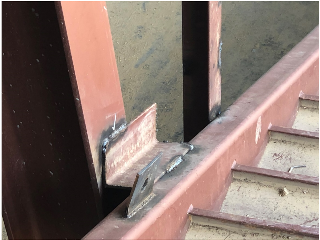
Figure 11 – Unsightly Weld at stair to structure (Assuming this is temporary)
