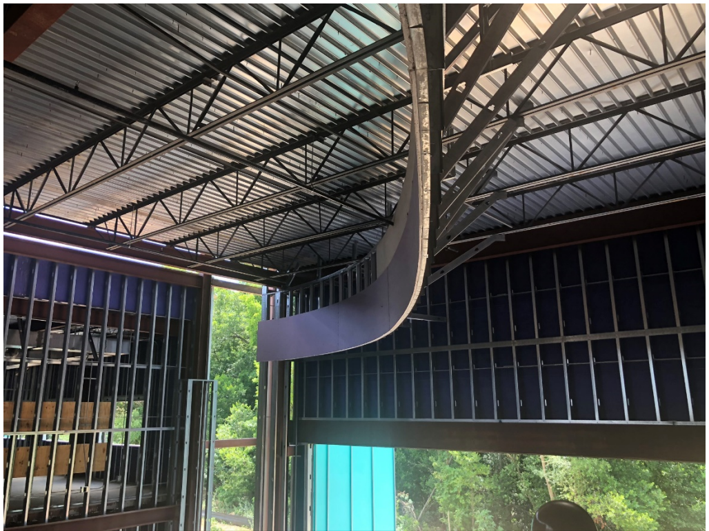
Figure 6 – Furr Down Curve Needs Attention (adjusting required at straightened portion)
