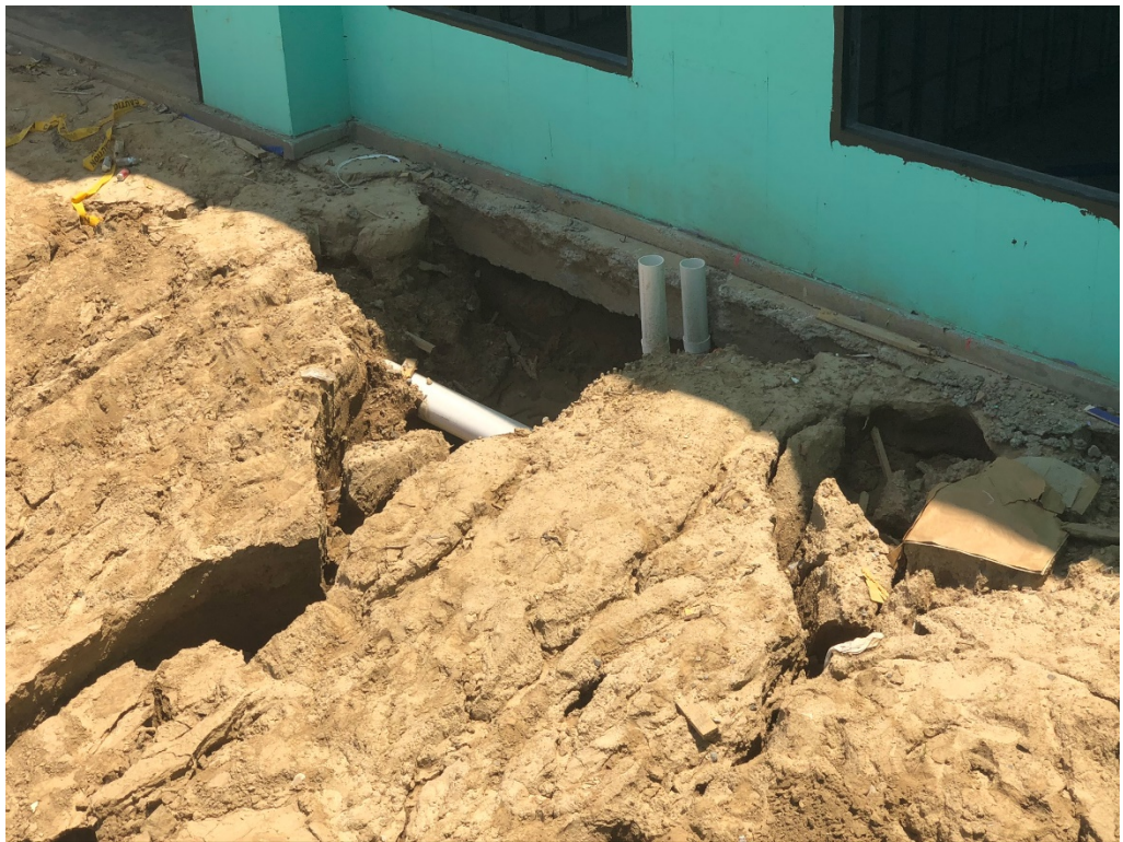
Figure 12 – West Elevation at North Structure Erosion
